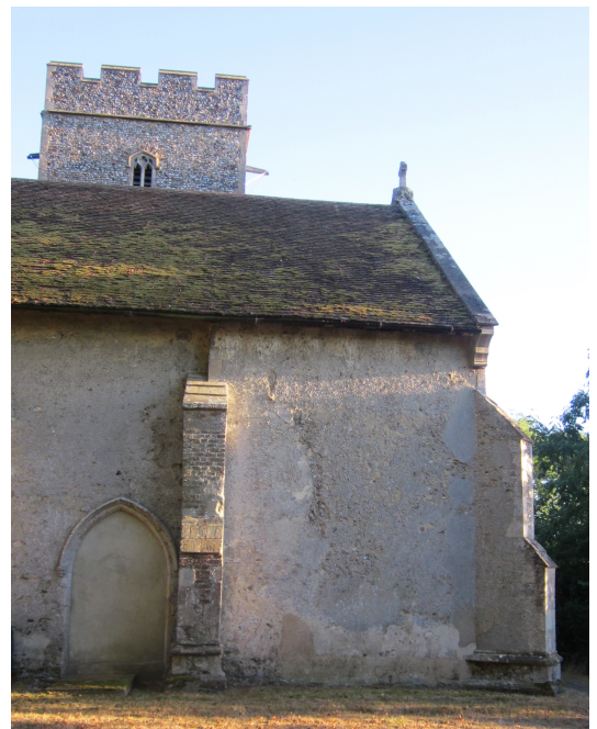
It can be seen that the nave was extended before the tower was built in c. 1400-20
